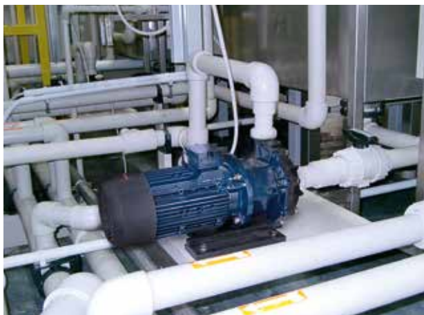
MAGSON BG 5 for circulating an electroplating bath with sulphuric acid via a heat exchanger to retain temperature.
