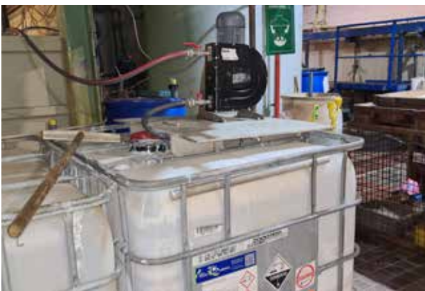
FHP 15: pumping 45 %, abrasive lime milk from a 1000 l IBC into a wastewater facility's receiver tank.
